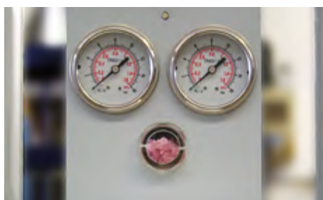
Pressure gauges & moisture indicators
